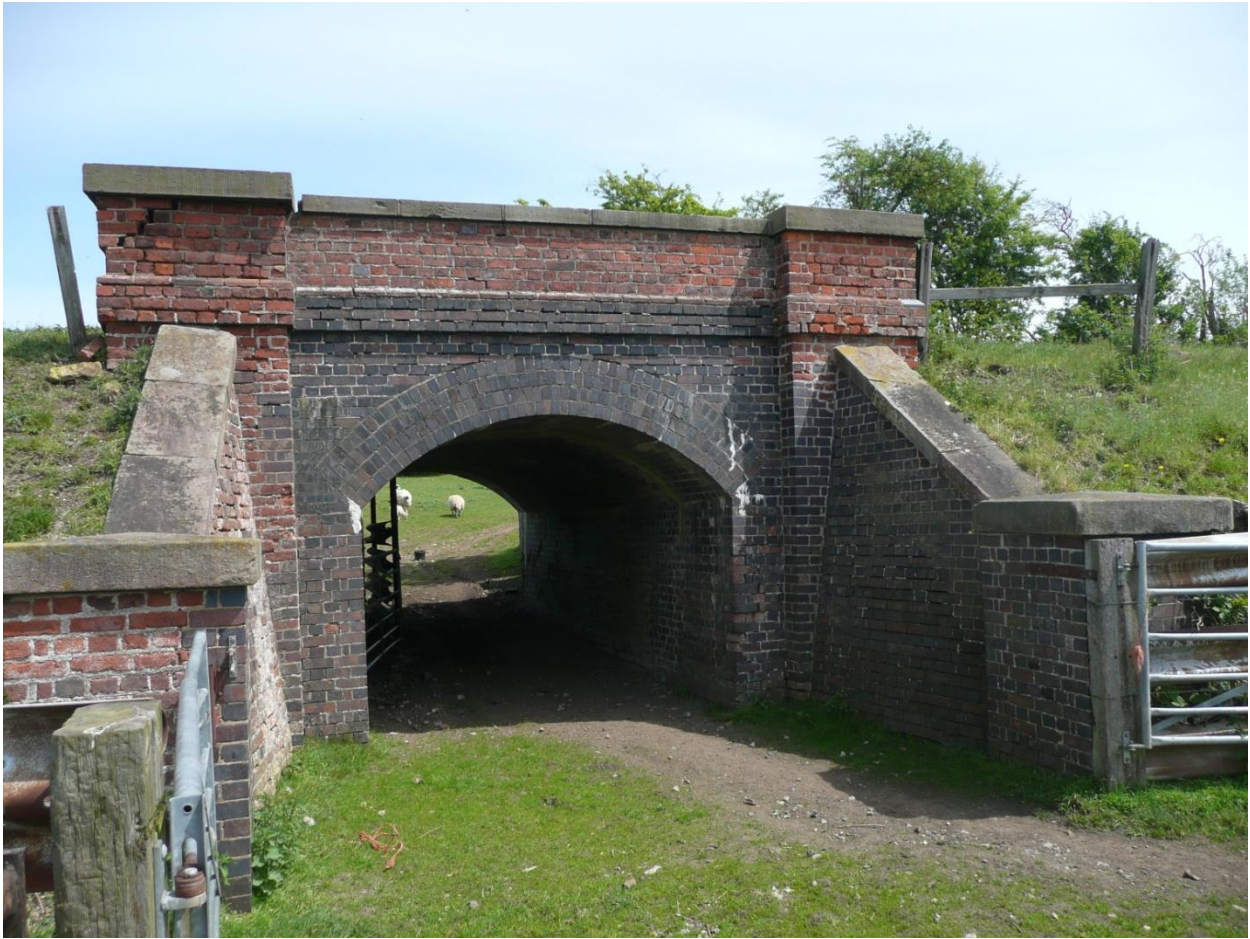
Bridge under the old London and North Western railway trackbed, near Twyford
